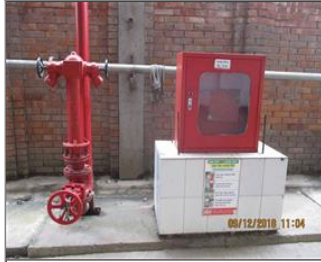
Photo of fire safety equipment Fire hose pipe.jpg
