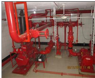
Photo of fire safety equipment Fire pump room.jpg
